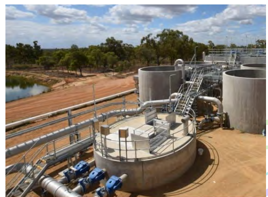
Above: Stage 1 – Upgrade of the Raw Water System and Water Treatment Plant.
